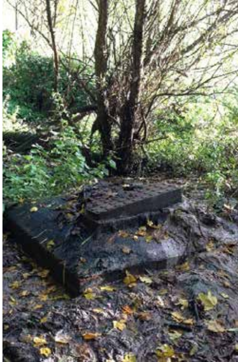
This image of a sewer overflow is the result of overstressed water infrastructure. One advantage of SuDS is their ability to remove surface water runoff from the sewer system, improving its capacity for managing wastewater.
